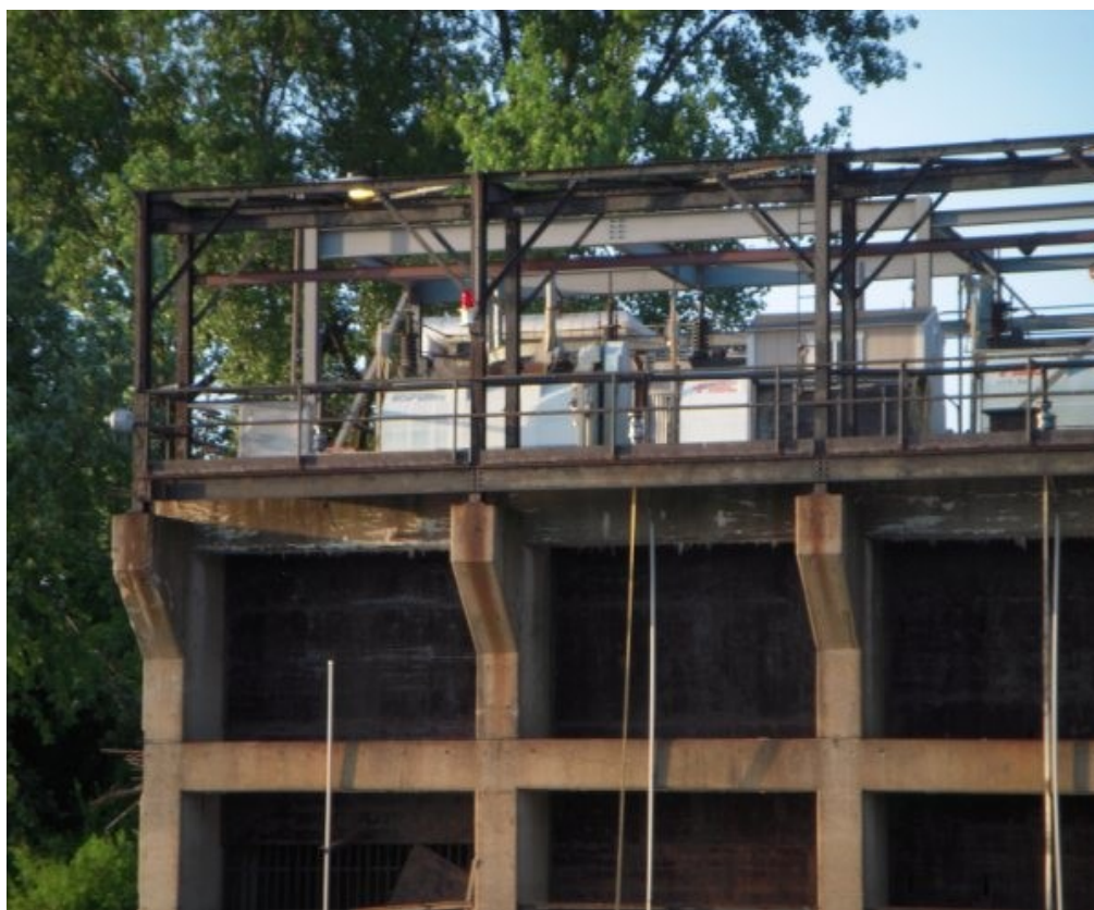
The water intake for the Illinois Power Company power plant near Alton Illinois
